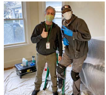
Jed Ader, Director of Facilities, and William Hopkins, Senior Maintenance Technician, prepare a room for a new resident.
